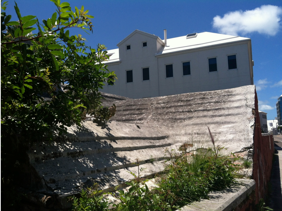
Figure 1.7: Like all traditional Bermuda roofs, Queen of the East's is stepped to collect fresh rainwater for use in the house. Photo by author, 2013.
